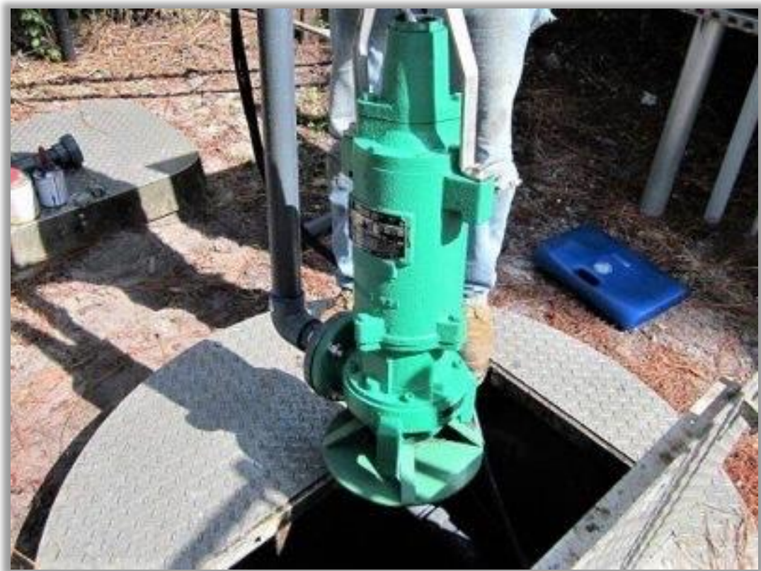
FLUSH: Key Pump Lifting
